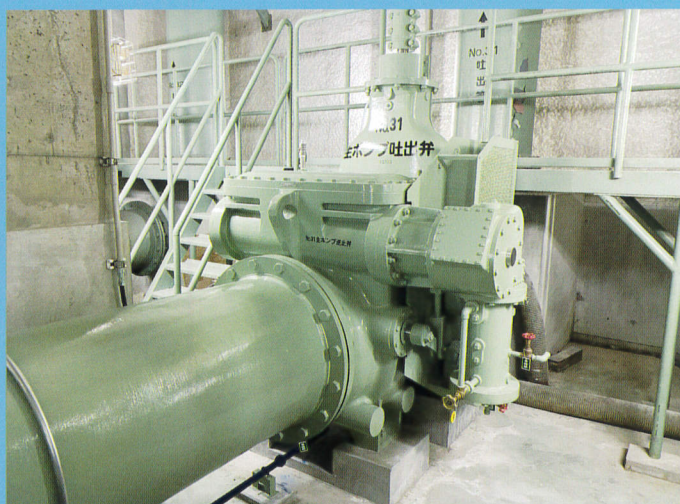
No.31主ポンプ吐出弁・逆止弁
